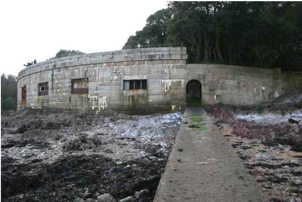
Garden Battery, Mount Edgecumbe. One of a series of fortifications built around Plymouth Sound during the 1860s as part of Viscount Palmerston's programme of defensive enhancements to Britain's naval bases. © details
