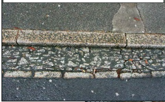
Good quality street surfaces in the upper parts of Church Street contrast with .....
